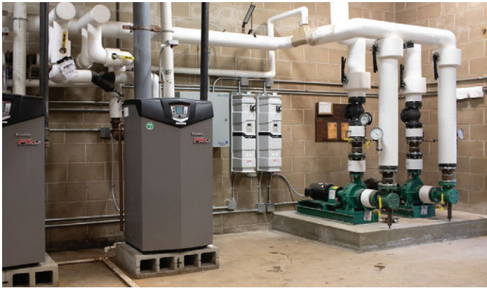
The City of Pawtucket's investment in building management systems helped to significantly reduce energy costs.
