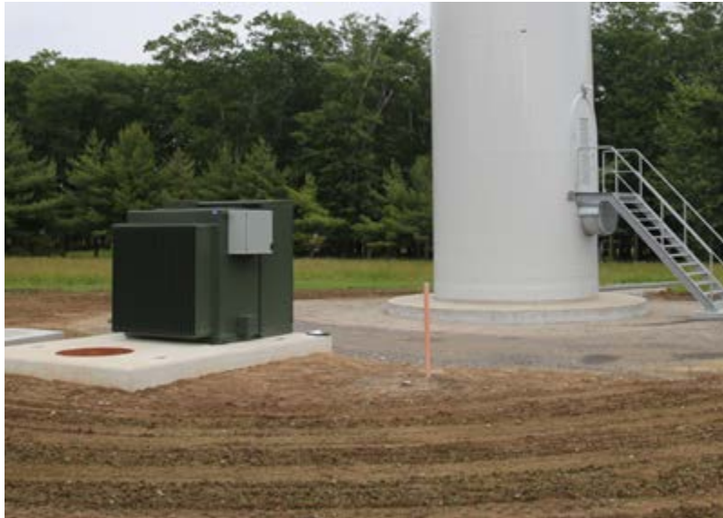
Figure 7. Base of Inspected Wind Turbine Generator and Pad-Mounted Transformer
